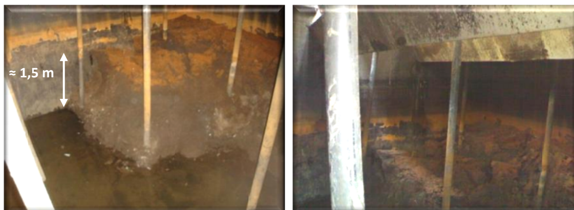
(a) Camada de areia no interior do reator UASB
