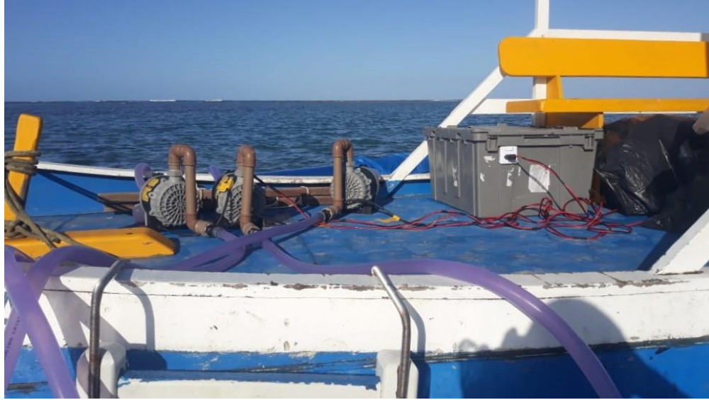
Figure 6 – Well pump connected to the watertight box, which presented a truck battery and a current inverter inside.
