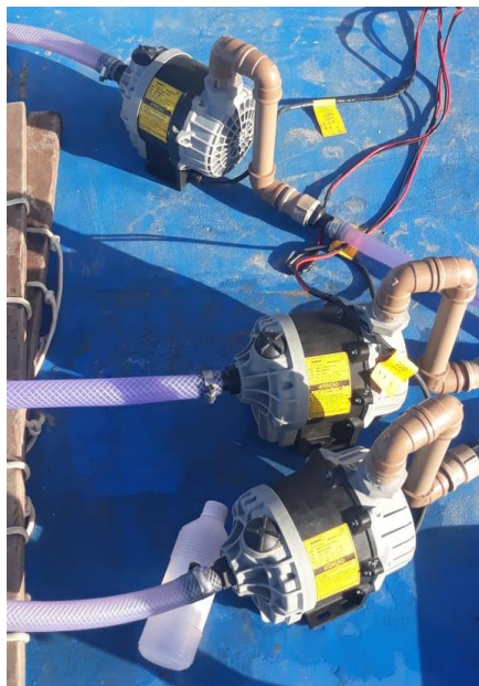
Figure 5 – Well pumps used during the experiment to fill and empty the pool.
